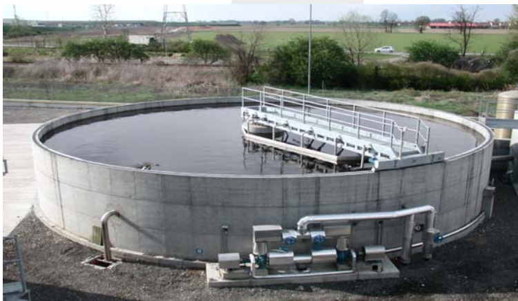
Settling and recycling
